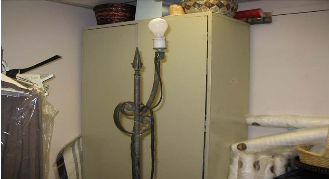
F1 – Fixture used as a trouble light
