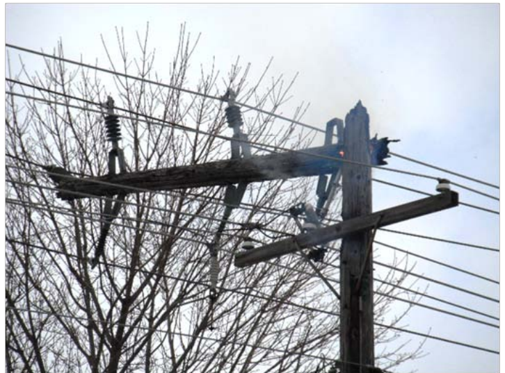
Image 9: Closer 'Before' photo of pole fire
