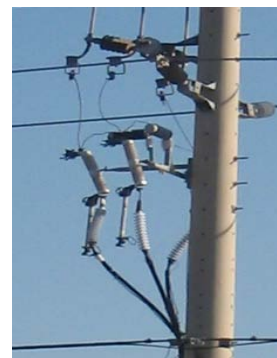
Image 3: Riser Cable Terminations
