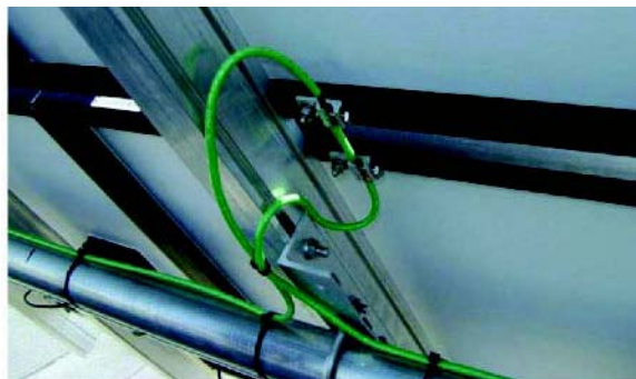
Photo B2 – Example of acceptable connection of bonding conductor
