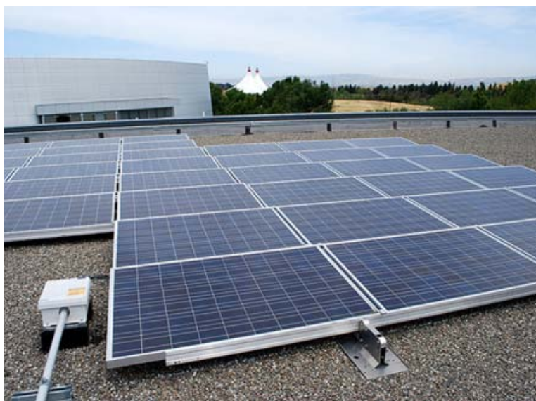
Photo B1 – Combiner box
