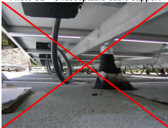
Photo B2 – Unacceptable cable support
