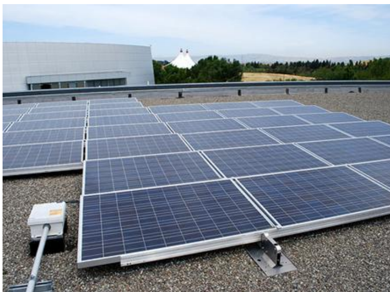
Photo B1 – Combiner box
