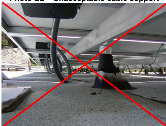
Photo B2 – Unacceptable cable support
