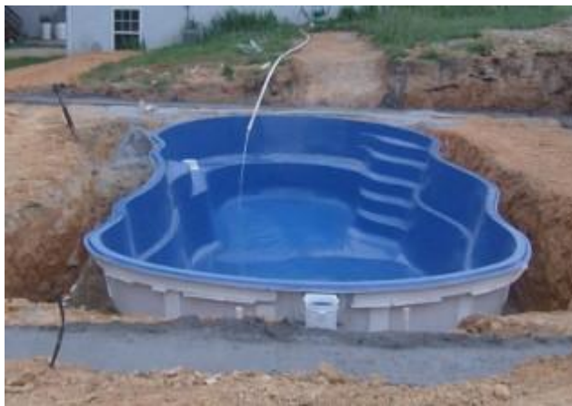
Photo B3 – Fibreglass pool
