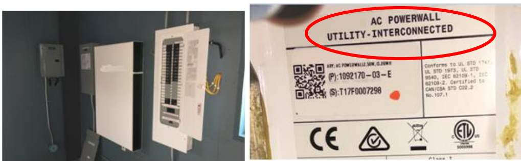
Photo B1 - Example of self-contained energy storage system and nameplate
