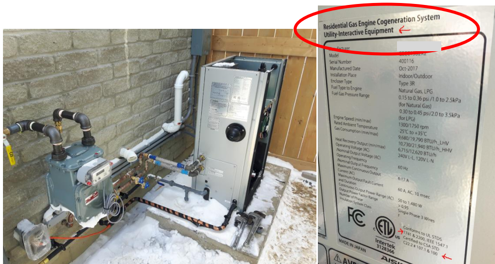
Photo B2 - Example of residential co-generation system and nameplate label
