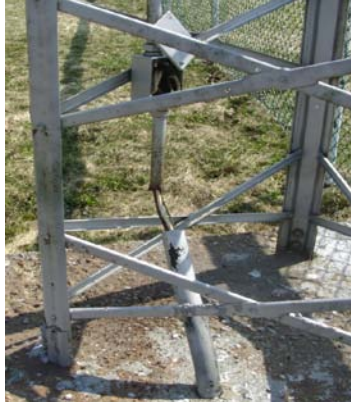
Photo F1 – Deteriorated and incomplete conduit system with exposed conductors
