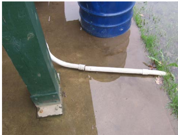
Photo F2 – Improperly protected conduit (Damaged)
