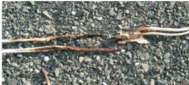
Photo F1 – Electrical equipment failure
