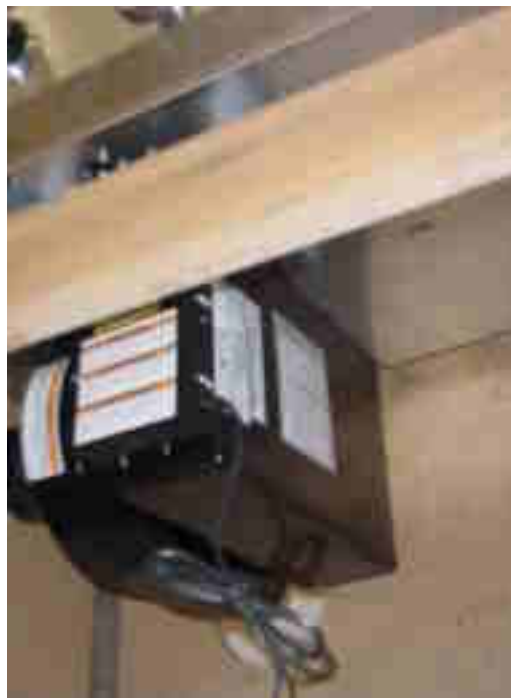
Vent Fan Housing Rating Plate (far left label)
