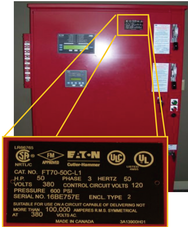
Figure 2: Affected Fire Pump Controller Serial Number Identification
